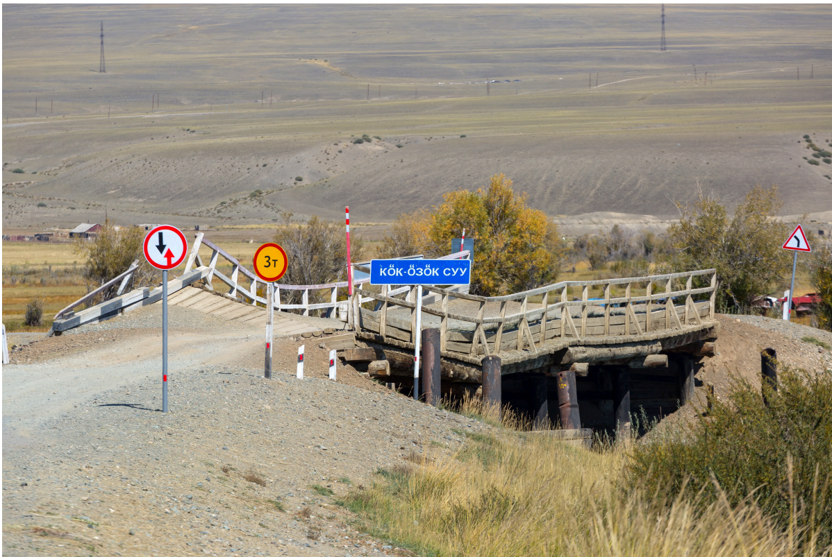
A bridge in the Altai Mountains, which turned “woozy” because of the melting permafrost. © 2021 Alexey Litvinov. All rights reserved.
